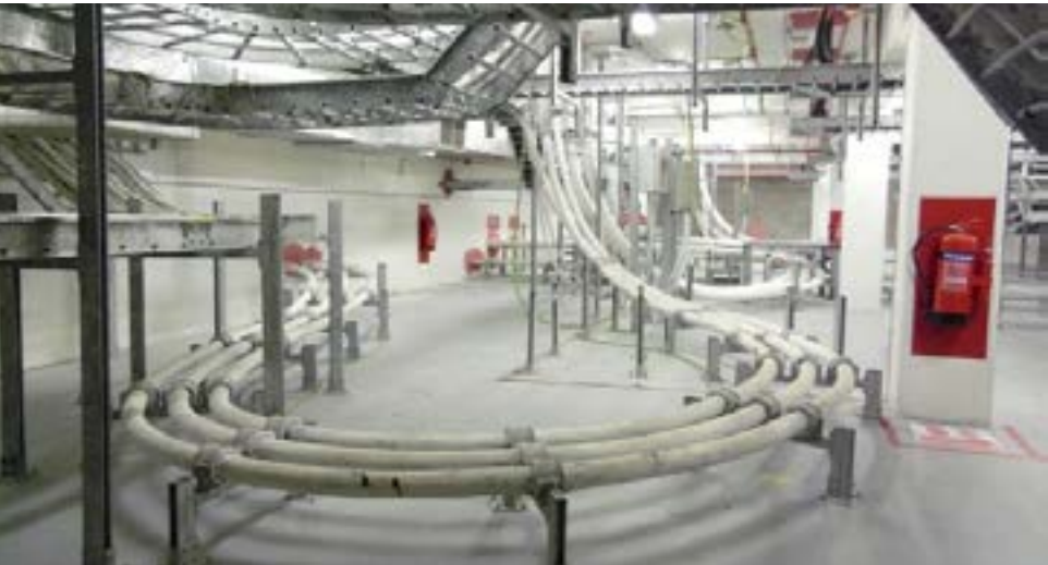
Project: West Buraydah 132/13.8 kV Substation Burayadh - KSA
