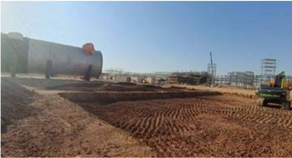
Project: Wa'ad Al-Shamal 132kV GIS Extension Wa'ad Al Shamal, KSA
