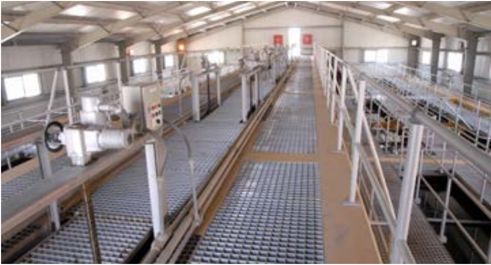
Project: Sewage Treatment Plant Quatif, KSA
