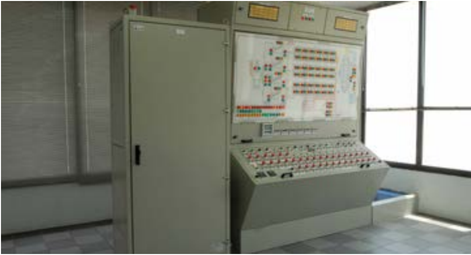
Project: Waste Water Treatment Plant Al-Khobar, KSA
