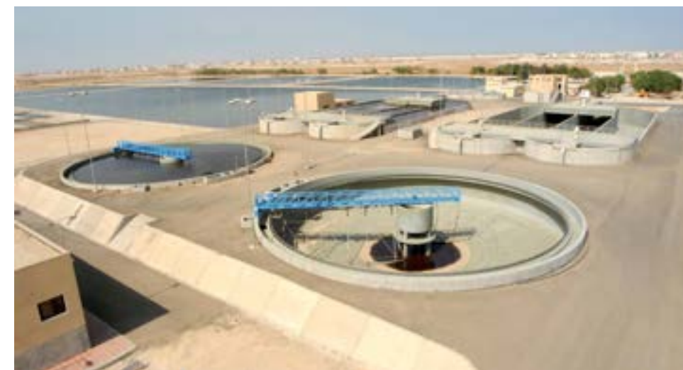
Project: Sewage Treatment Plant
