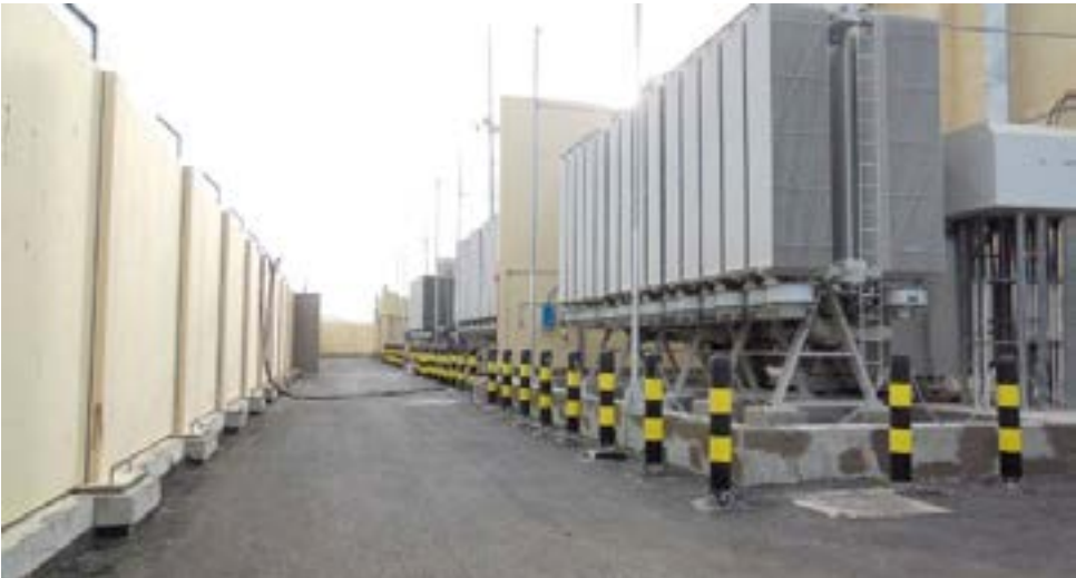
Project: West Buraydah 132/13.8 kV Substation Burayadh - KSA
