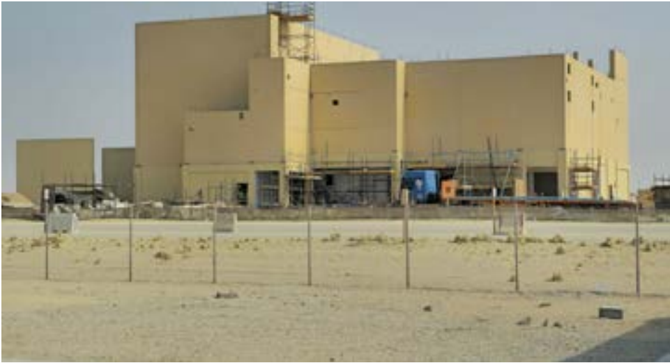
Project: EPC GIS Substation (Phosphate 3/Phase 1) - RAK Ras Al-Khair, KSA
